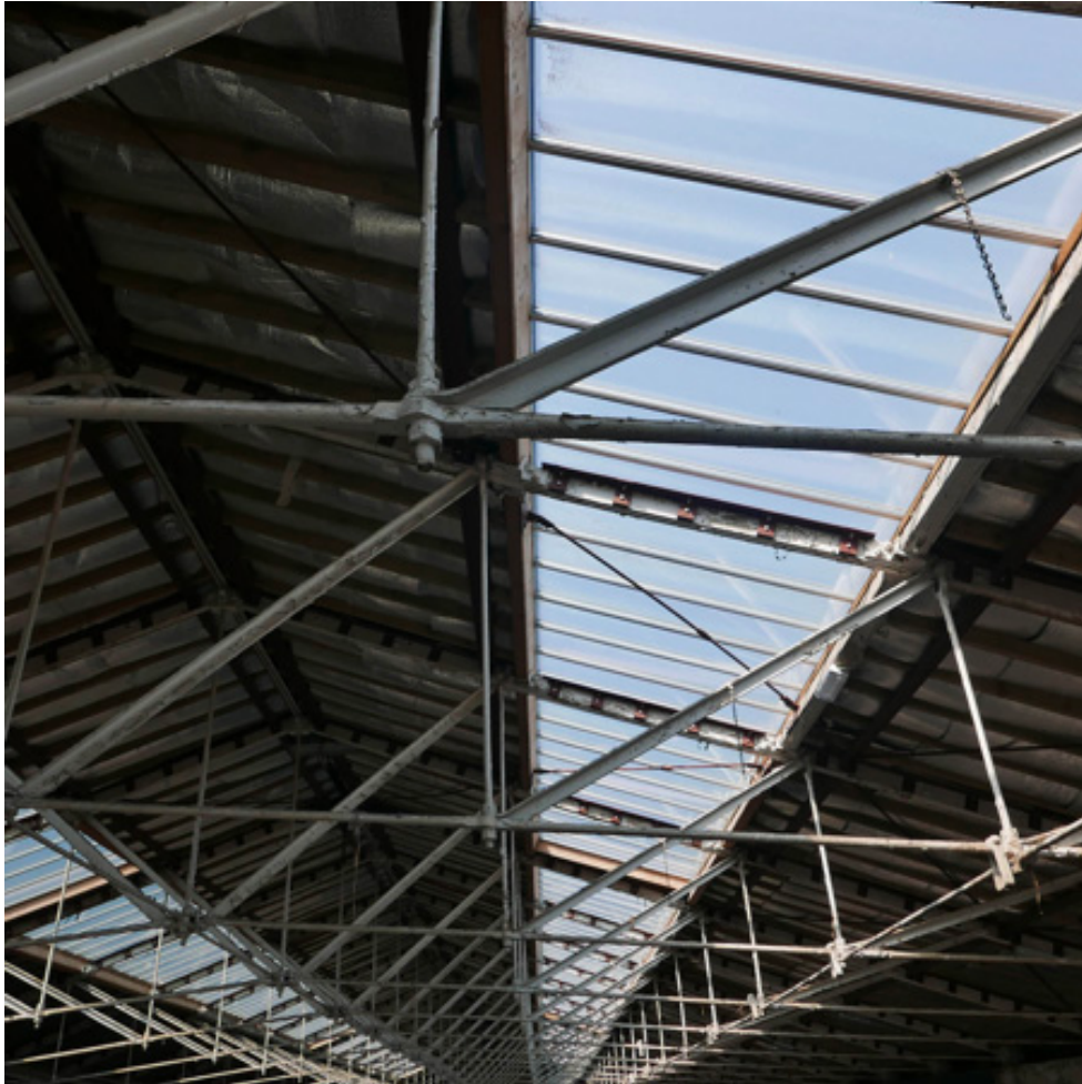
Reasonably light work can be suspended from metal rafters. They are not too high to reach easily.
